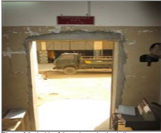
Photo of the inside of the main production hall Emergency Exit.JPG
