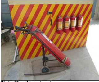
Photo of fire safety equipment Fire Extinguishers.JPG
