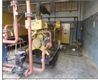
Photo of the inside of the main production hall Generator Area.JPG
