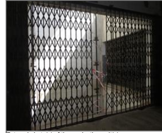
External photo(s) of the production unit(s) Cargo Lift With Interlocking System Installed.JPG
