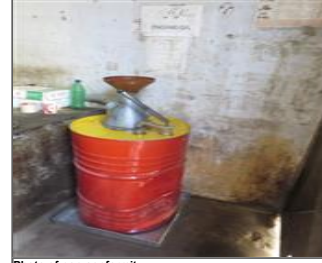
Photo of non-conformity Engine Oil With Secondary Containment But Without MSDS.JPG
